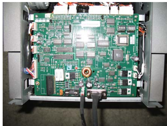
Power and communication cables
